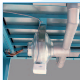
Ventilator for air supply
